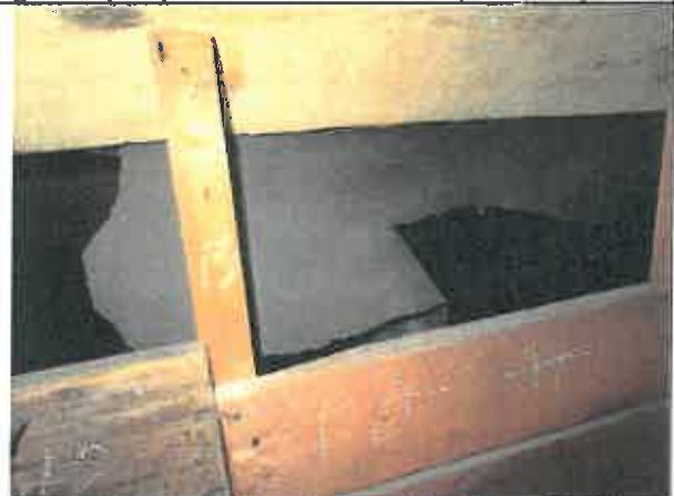
Photo 15: Tar paper observed in Room 28 (Non-Asbestos).
