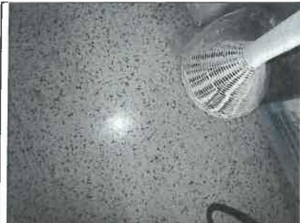
Photo 13: 8" floor tile (Type D— white with red and green spots) observed in Room 20 (Asbestos).
