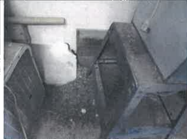
Photo 21: Vermiculite insulation observed within the walls in Room 36 (Asbestos).
