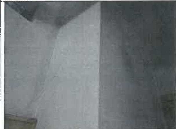
Photo 3: Plaster observed in Room 1 (Asbestos).
