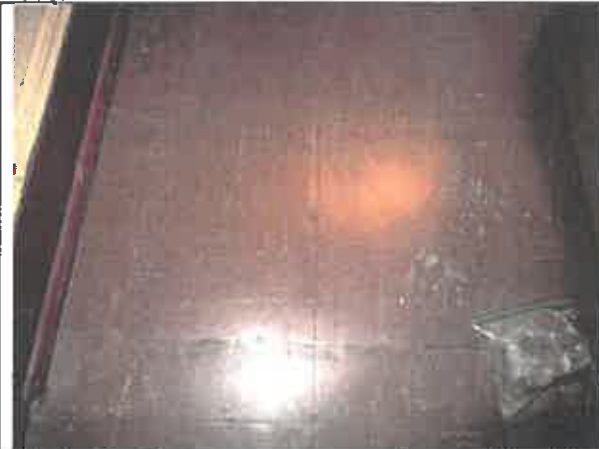
Photo 19: 8" floor tile (Type G— brown with white streaks) observed in Room 33 (Asbestos)
