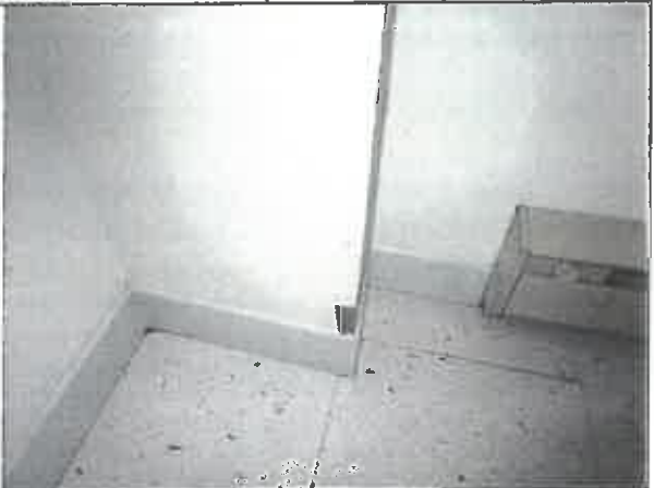
Photo 6: Drywall joint compound observed in Room 5 (Asbestos).
