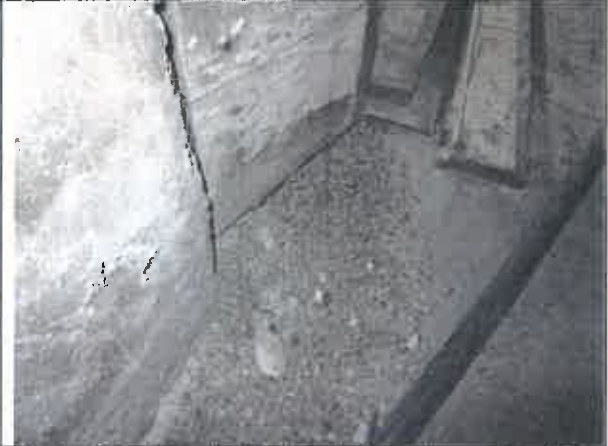
Photo 22: Vermiculite insulation observed within the walls in Room 38 (Asbestos).
