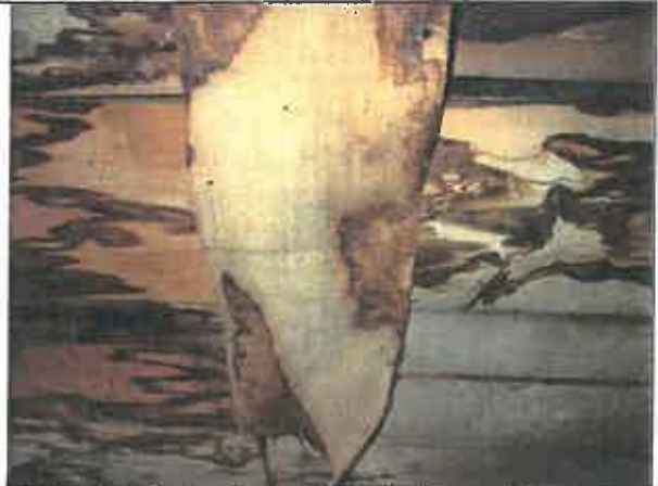
Photo 16: Burlap-like material observed in Room 28 (Non-Asbestos).
