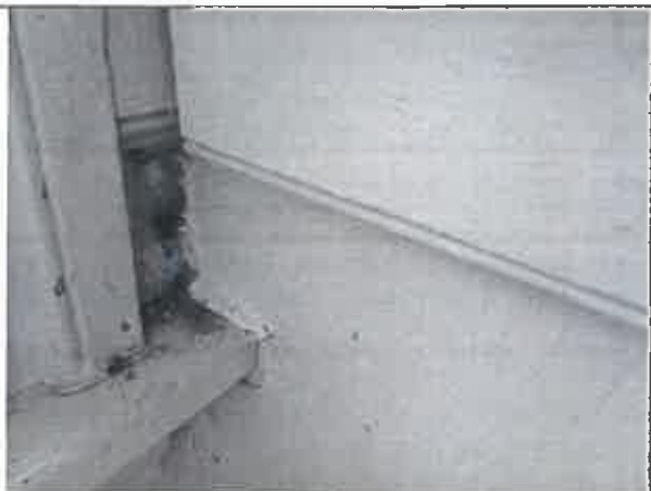
Photo 8: Burlap-like material (Type A) observed on lower wall portion of Room 15 (Non-Asbestos).
