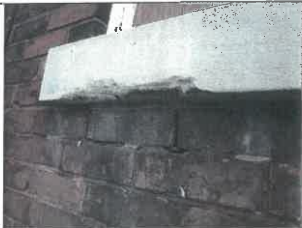
Photo 2: Window caulking (Grey) observed on the building's exterior (Asbestos).
