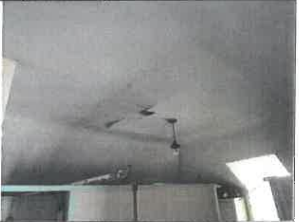
Photo 18: Plaster observed in Room 27 (Asbestos).
