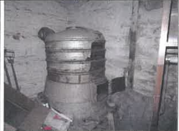
Photo 24: Boiler insulation observed in Room 38 (Asbestos).
